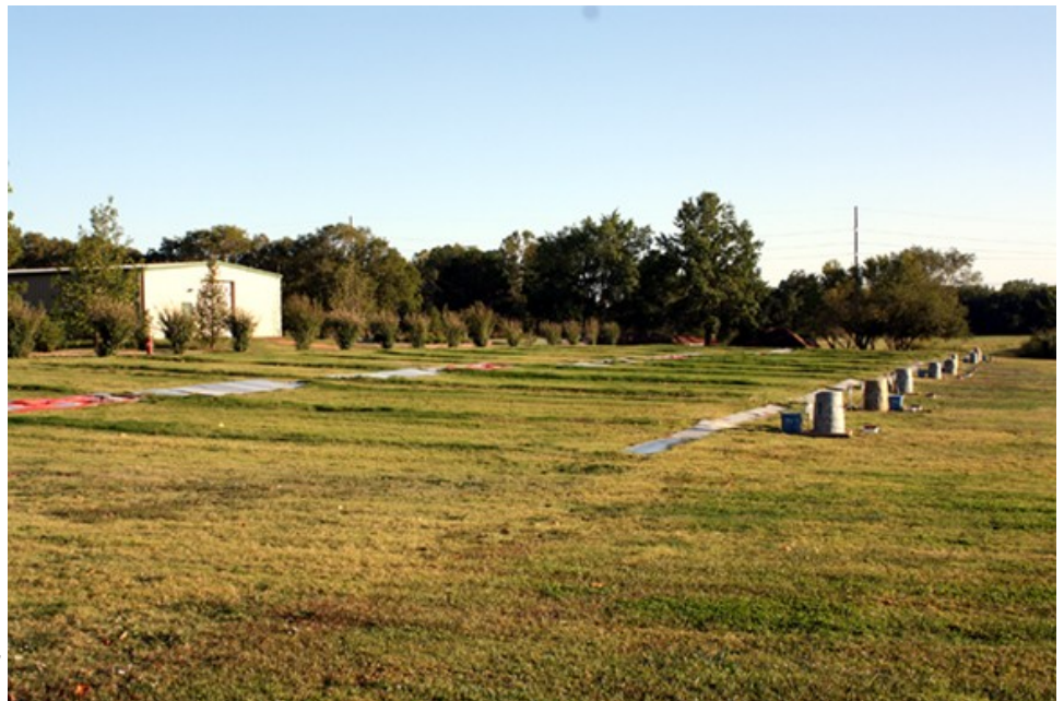
Figure 1. The OSU Turfgrass Research Runoff Site following construction of the filter system in the middle of each plot.
