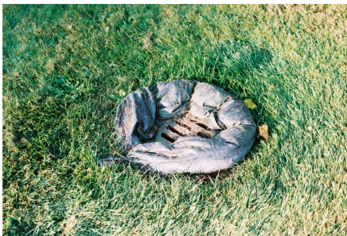
Figure 2. Filter socks were installed around each inlet within the eastern drainage area. The filter socks were filled with 75% steel slag, 2.5% cement kiln dust (CKD), and 22.5% silica sand by volume.
