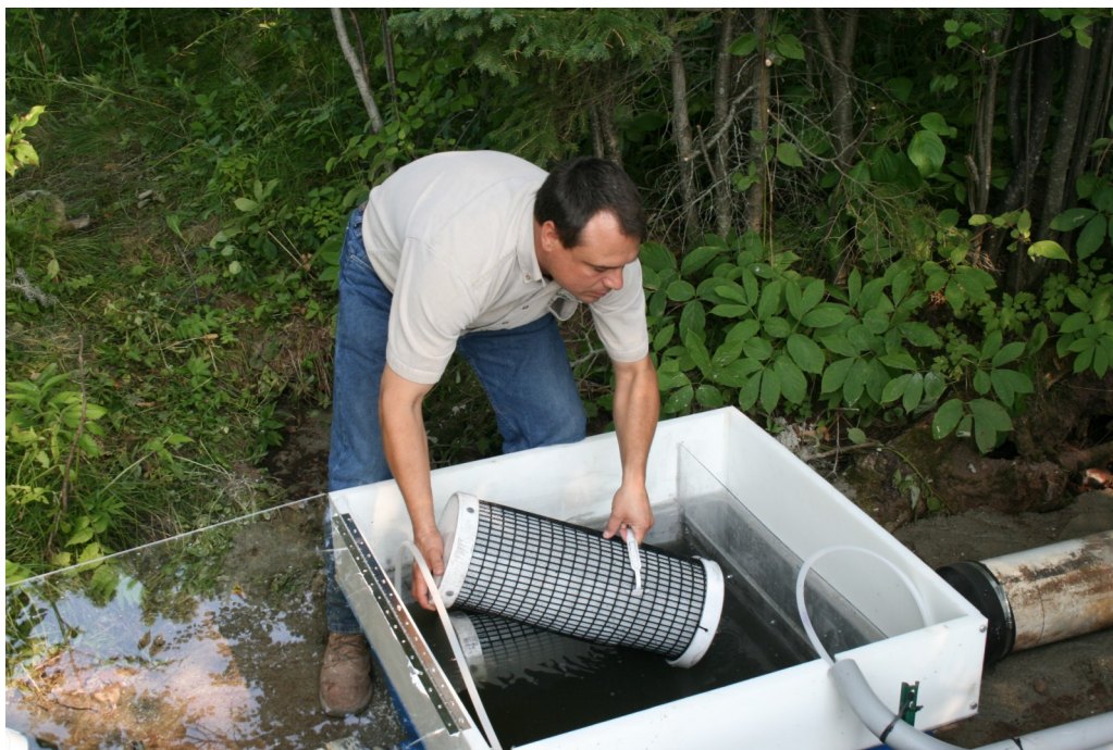
Figure 1. Filter cartridges are being evaluated for filtering phosphorus from leaving a golf course property.
