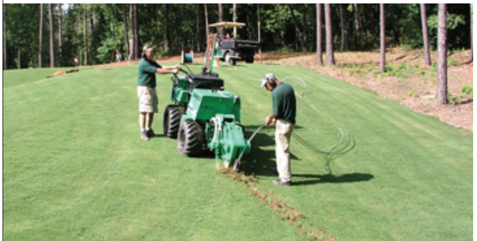
Wire materials and installation are the most expensive costs for a fan project. Installing the wire to the proper depth and according to local electrical codes is essential to supply consistent power to fans.
