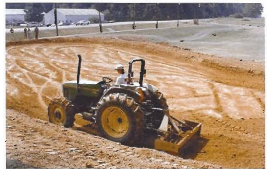
The extra time spent preparing the subgrade will result in a smooth, well-compacted base on which to build the remainder of the green.
