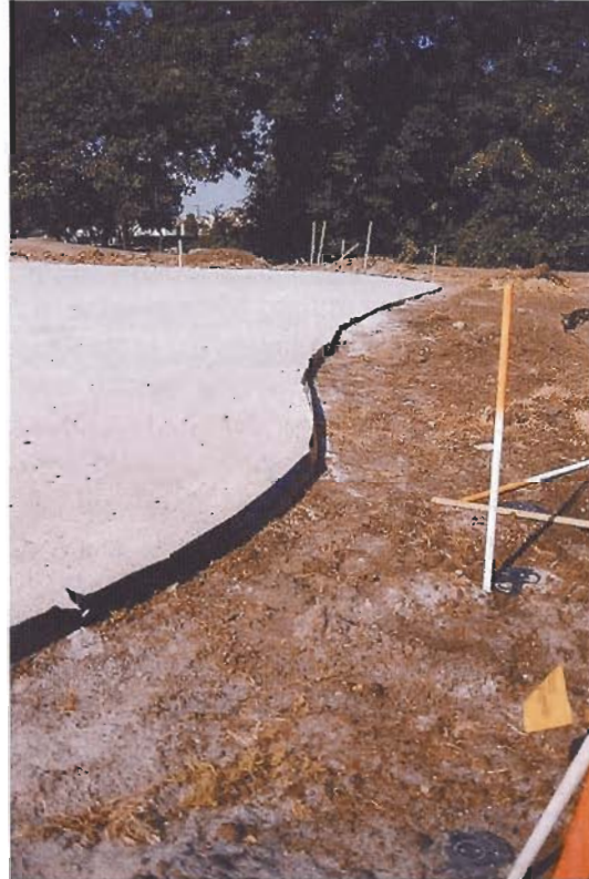
Notice that approximately four inches of the barrier has been left above the surrounding grade to help prevent soil from the surrounds from washing onto the green. It is removed later with a carpet knife or similar tool.
