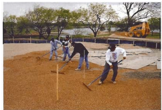
The gravel should be spread to a minimum depth of four inches and according to the grade stakes. The surface of the gravel layer should “mirror” the finished surface of the putting green.
