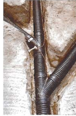
Lay a #14 irrigation wire in each ditch to allow easy location at a later date using a wire tracking device.
