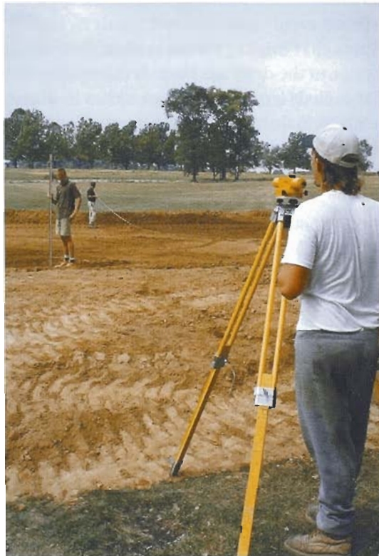
Use a surveying instrument to ensure the drainage ditches have at least 0.5% slope to the exit points.
