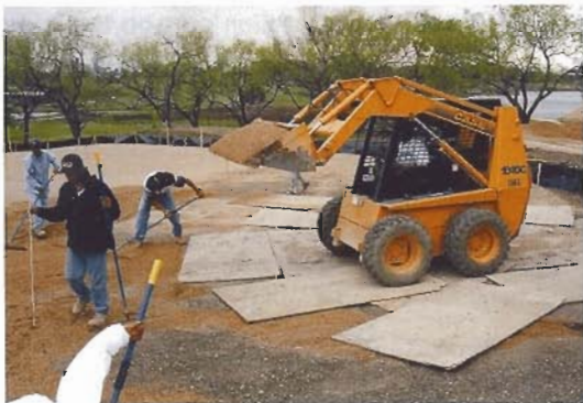
Heavy plywood is used to prevent damage to drainage lines from heavy equipment.
