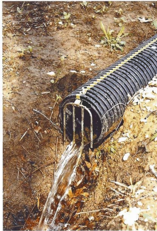
The end of drainage lines must be protected to prevent animals from entering the pipe.
