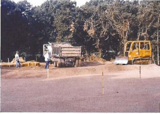
Spreading and dumping equipment should remain on the rootzone mixture instead of the gravel to avoid damage to the drainage system.
