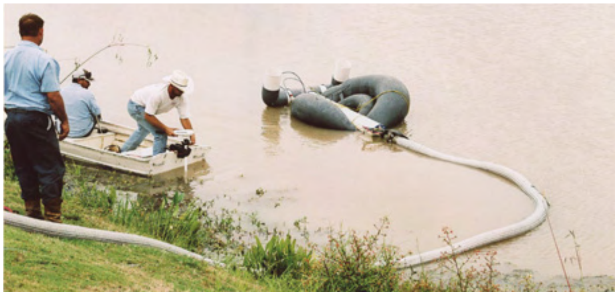
This photo shows the installation of a submersible diversion pump so another structure is not seen on the golf course. The maintenance of submersible pumps is not difficult.
